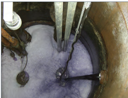
3.5m (11ft) FOAMY WET WELL PUMP CONTROL
