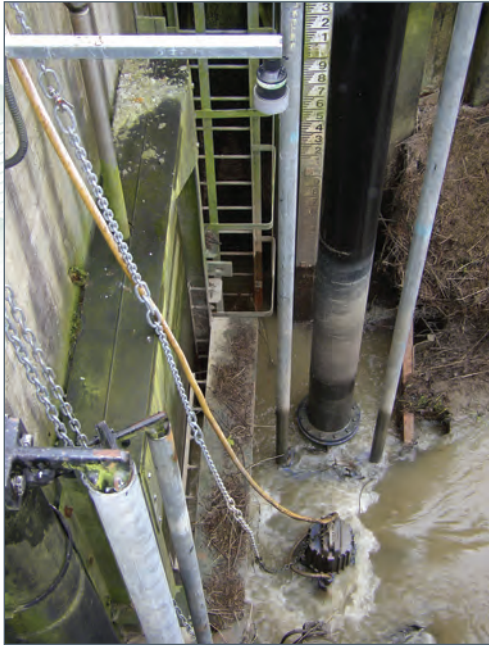
7m (23ft) PUMP CONTROL
